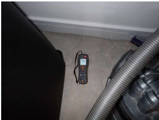
High moisture understairs cupboard
