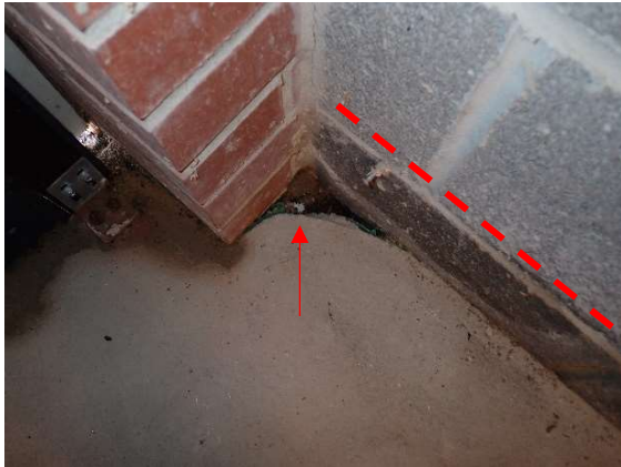
Floor dpm not lapped with wall (red arrow) Red dotted line shows level of wall dpc.
