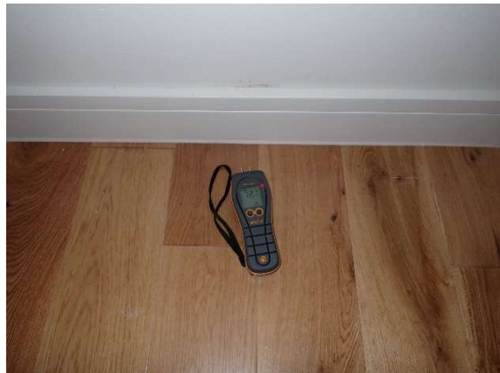
Deterioration and high levels of moisture on partition
